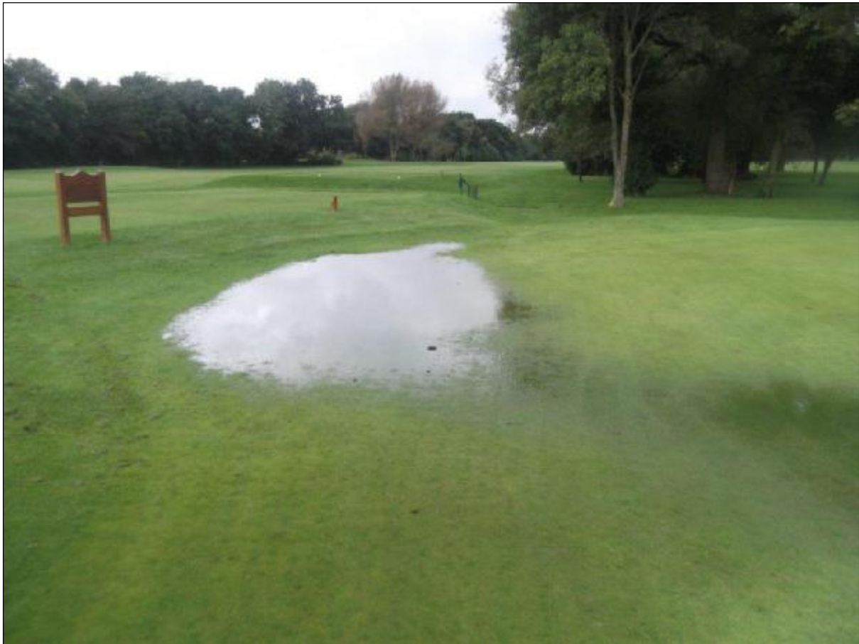
Photograph 3 – Persistent wet area located through the left hand side of the 9 th green.
